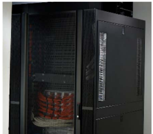
Installed on AR3340 enclosure
